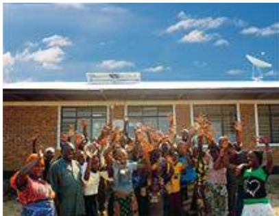
Solar modules installed at a school (Tanzania)
