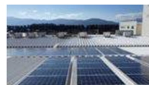
■ Nagano Okaya Plant (173kW) (introduced in FY2011 and expanded in FY2014)
