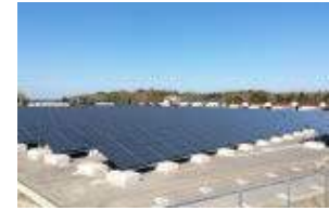
■ Former Chiba Plant site (688 kW) (introduced in FY2015)
