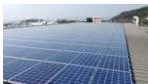
■ Shiga Gamo Plant (571kW) (introduced in FY2011 and expanded in FY2013 and FY2015)
