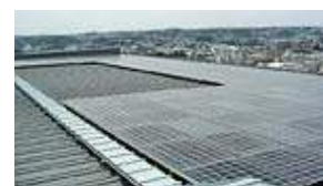
■ Yokohama Office (58kW) (introduced in FY2012)
