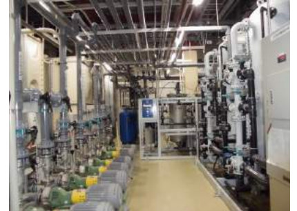
Wastewater recycling equipment
