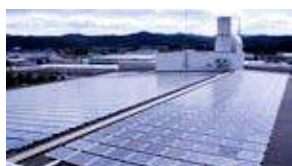
■ Hokkaido Kitami Plant (615kW) (first introduced in FY2011 and expanded in FY2017)
