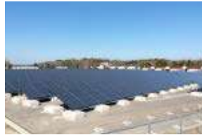
■ Yamagata Higashine Plant (688kW) (introduced in FY2015)
