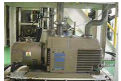
Vacuum pump with inverters
