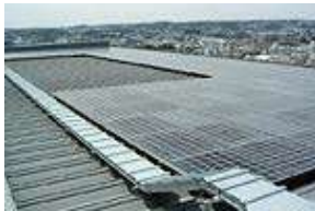
■ Yokohama Office (58kW) (introduced in FY2012)
