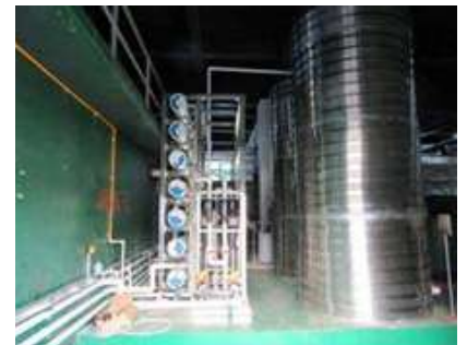
Wastewater Recycling Equipment
