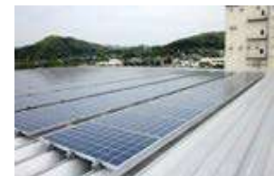
■ Kagoshima Sendai Plant (949kW) (introduced in FY2011 and expanded in FY2014 and FY2017)
