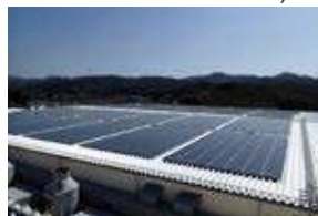
■ Kyoto Ayabe Plant (1,843kW) (introduced in FY2014 and expanded in FY2016 and FY2017)
