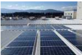
■ Nagano Okaya Plant (173kW) (introduced in FY2011 and expanded in FY2014)
