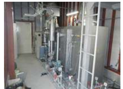
Waste heat boilers
