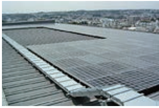
■ Yokohama Office (58 kW) (introduced in FY2012)
