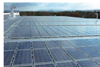
■ Shiga Gamo Plant (141 kW) (introduced in FY2011)
