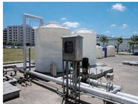
Water storage tank
