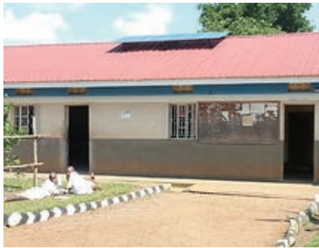
Solar modules installed on a school (Uganda)
