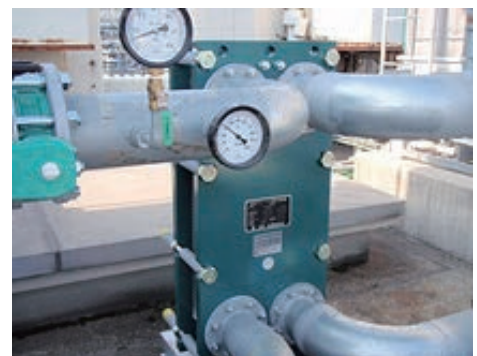
Heat exchanger (Shiga Yasu Plant)
