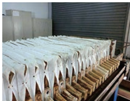
Sludge water-extraction machine
