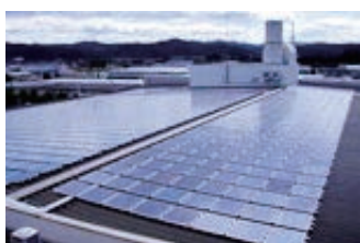
■ Hokkaido Kitami Plant (115 kW) (introduced in FY2011)
