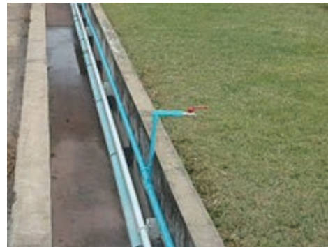
Piping used for watering
