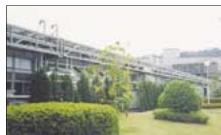
Moving underground pipes overhead (Kagoshima Kokubu Plant) allows for easy visual inspection and leakage detection.
