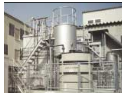
Denitrification processing facility (Shiga Yohkaichi Plant)
