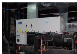
Waste-heat-recovery heat pump/chiller units
