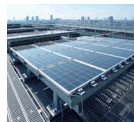
Solar power generation system installed on the roof
