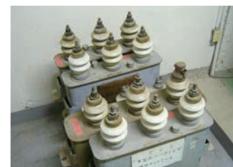
PCB waste storage area (Kagoshima Sendai Plant)
