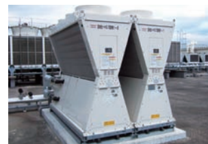
High-efficiency heat pumps (Shiga Yohkaichi Plant)
