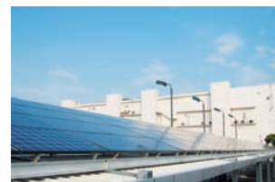
Solar Photovoltaic System set up on the roof of the parking lot for bicycles
