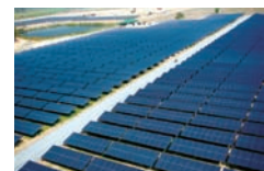
Solar Power Generation System installed in the city of Korat, Thailand
