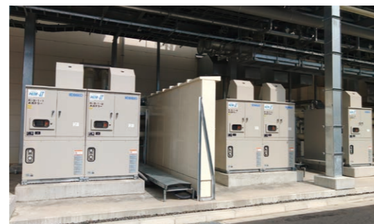
Kyoto Ayabe Plant: Exhaust heat recovery
